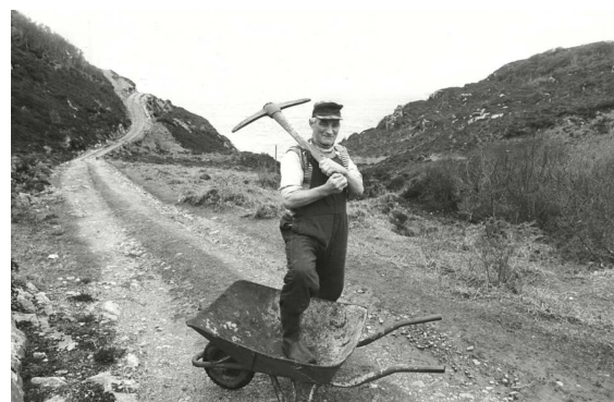
Figure Raasay 1.14: Calum MacLeod, armed with pick-axe and wheelbarrow during the construction of the Brochel to Ardnish road.
