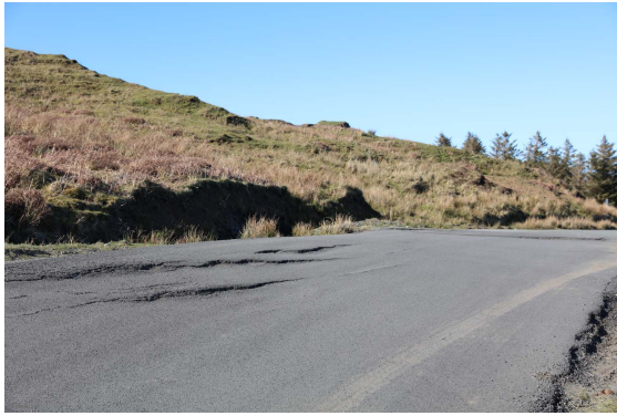
Figure North Skye 9.27: Tension gashes on the public road at Flodigarry due to landslip-induced movement.
