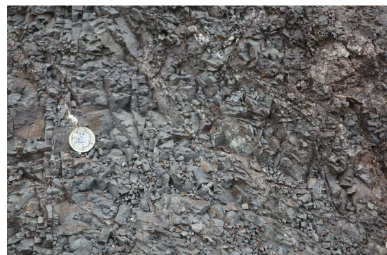
Figure West Skye 4.7: Detail of volcaniclastic shales with mineralised, close-spaced joints, at Greep. Coin c. 24mm across.
