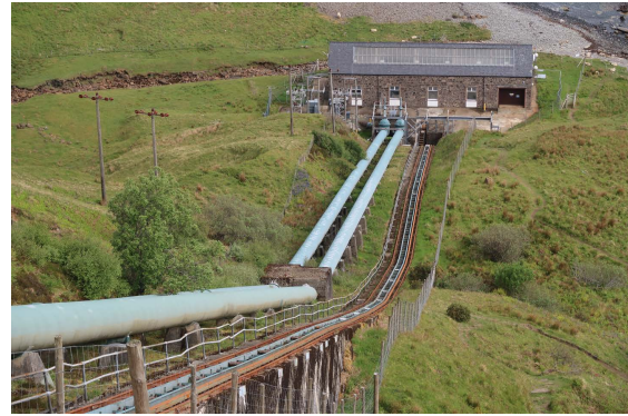
Figure North Skye 2.6: Twin pipes of the Storr Lochs hydroelectric scheme.
