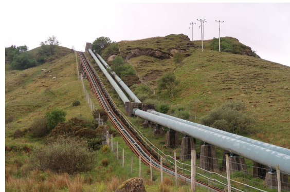
Figure North Skye 2.7: Twin pipes of the Storr Lochs hydroelectric scheme.
