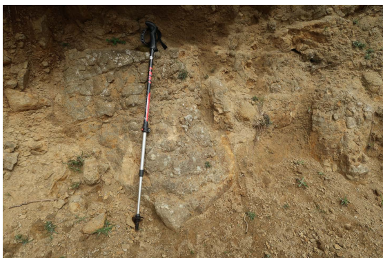
Figure North Skye 12.17: Thoroughly weathered and degraded sill rock at Peingown. Pole c. 1m long.
