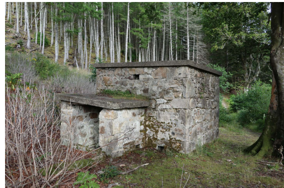
Figure Raasay 4.18: Storage building for explosives, north side of track, east of Mine #2 site.
